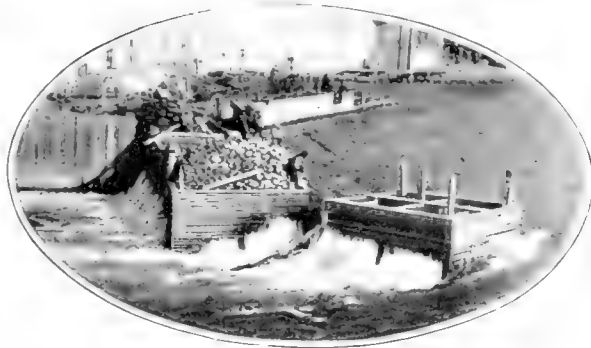
If a cable should snap, the crib would be dashed to pieces on the rocks below the falls
